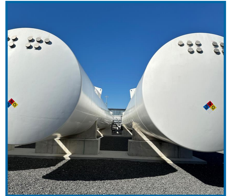
380M 3 Liquefied Natural Gas Storage Tanks
