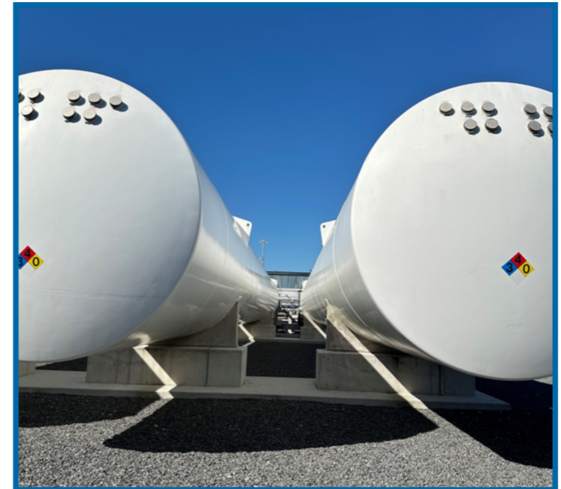
380M 3 Liquefied Natural Gas Storage Tanks
