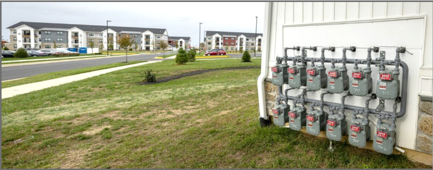
In Middletown, DE we have added 10+ multifamily buildings, representing over 350 units in the last few years.
