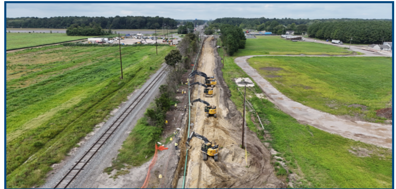
Diggers at work on an Eastern Shore Natural Gas reliability project in Salisbury, MD
