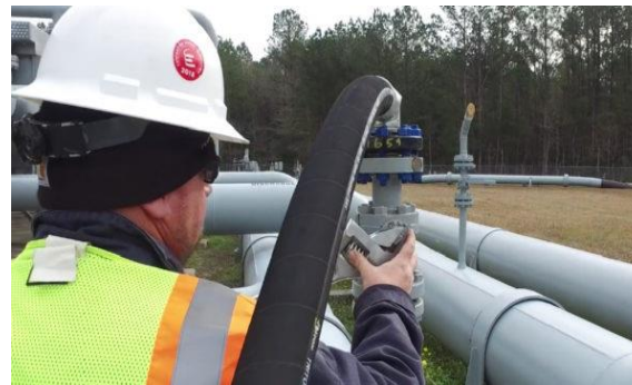
Utility Gas Supply Services
